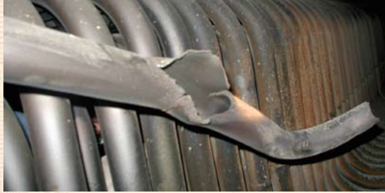
(photo at left) A ruptured boiler tube gives an indication of the pressure and heat to which the tubes are subjected
