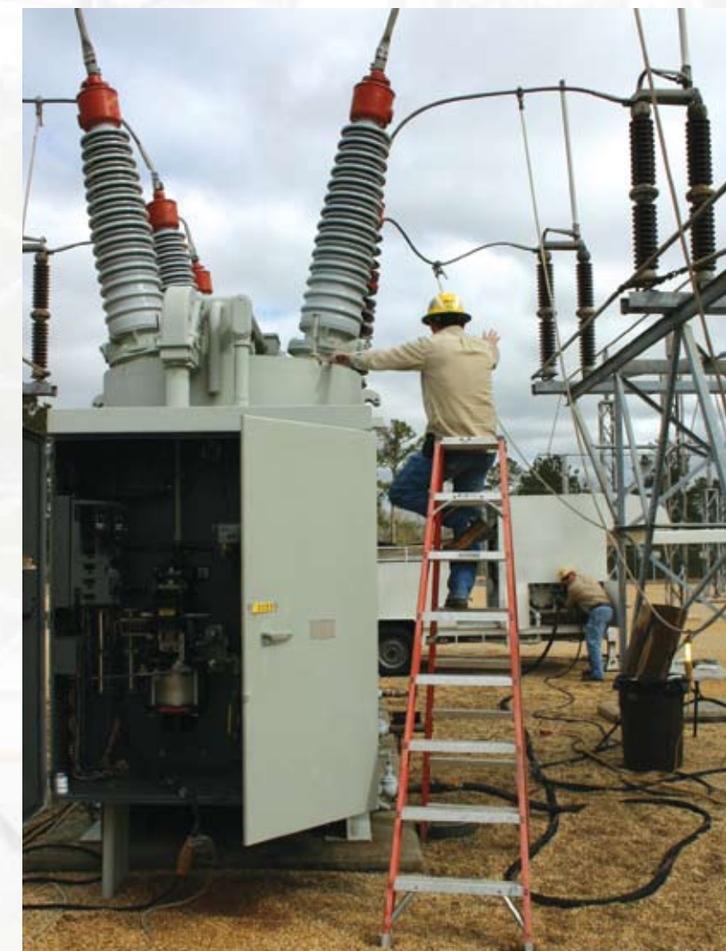
Technicians Josh Beech (on ladder) and Matt Simpson refill the oil on a 161kV breaker at Columbia
