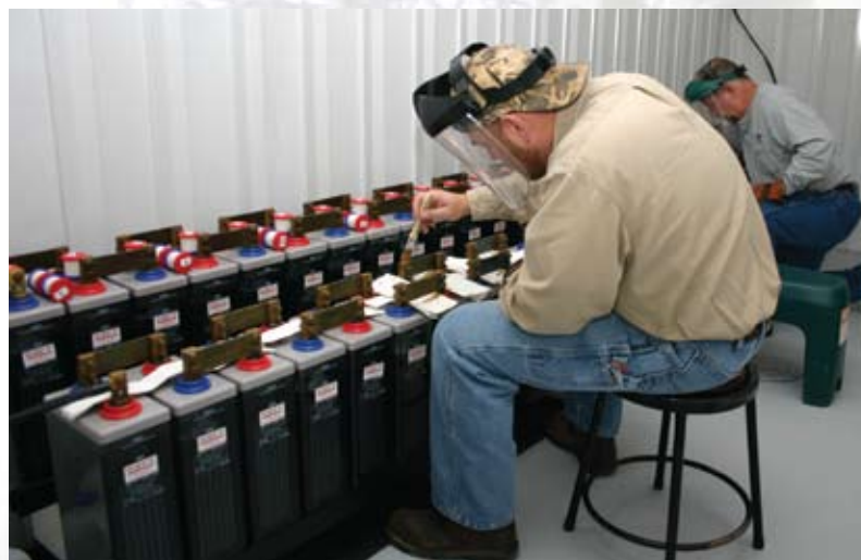
Technicians Matt Simpson and Kenny Casanova perform battery maintenance at Waynesboro
